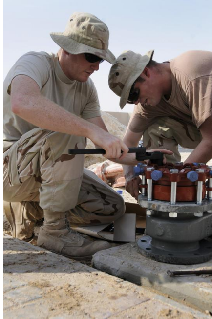
Figure 6.16: A mega lug is being prepared as a temporary valve to close off the end of a broken water pipe in order to restore water to the Blatchford-Preston Complex 56
