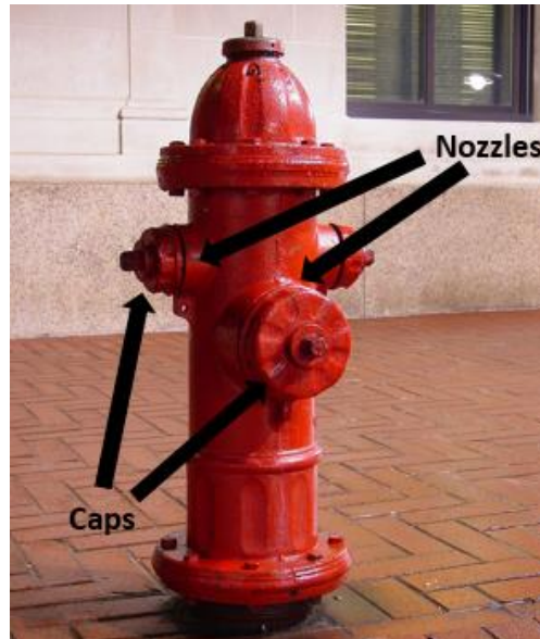
Figure 8.6: The caps and nozzles of a fire hydrant 83
