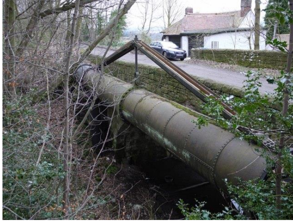
Figure 6.4: An example of a grey cast-iron pipeline 43
