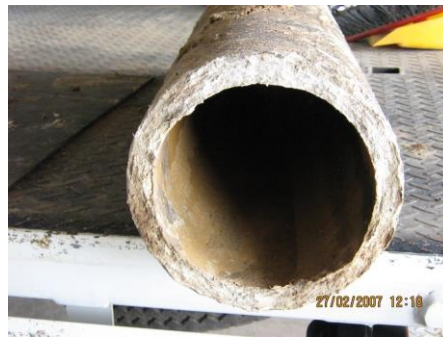
Figure 6.8: A brittle Asbestos-cement pipe 47
