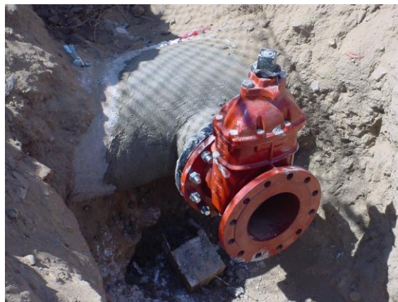
Figure 7.5: A below-ground gate valve 61
