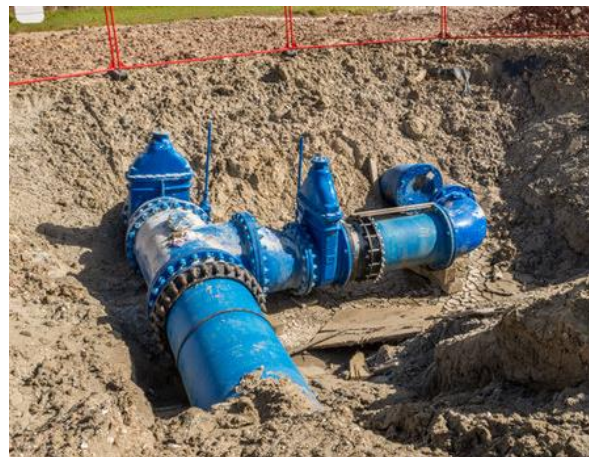
Figure 6.13: An exposed water main joint 53
